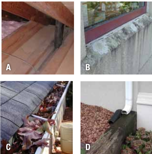
Figure 8. Sources of moisture around and in structures include, but are not limited to, (A) collection of water in attics from leaky pipe penetrations on the roof, (B) collection of water behind improperly installed siding around windows (note growth of lichens, indicating excessive moisture accumulation), (C) leaf-clogged gutters, and (D) downspout exhaust too close to the structure.
