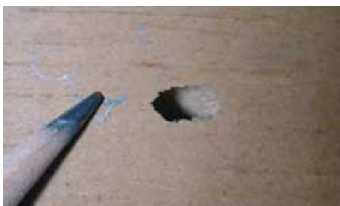
Wood-boring beetle exit hole
