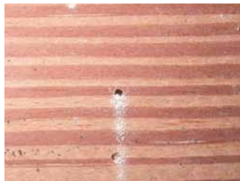
Anobiid powderpost beetle exit holes in an infested crawlspace joist.
