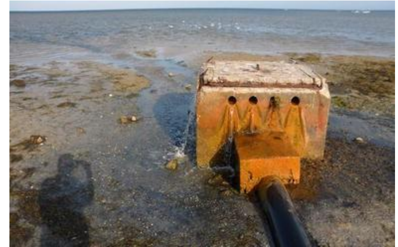
Sewage Treatment Plant Discharge
